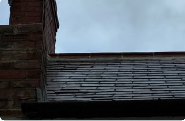
Flashing around chimney shows wear
