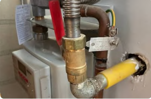
Corrosion visible on gas pipe
