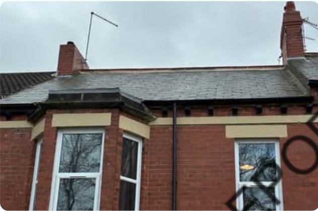
Moss and algae on roof tiles
