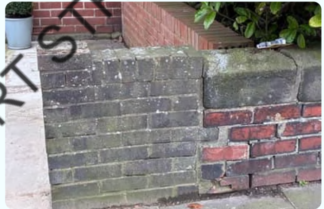
Damaged bricks and mortar loss
