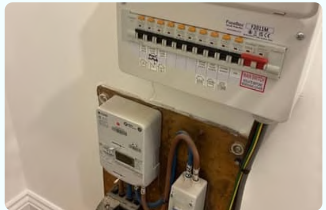
Electrical panel mounted on timber board
