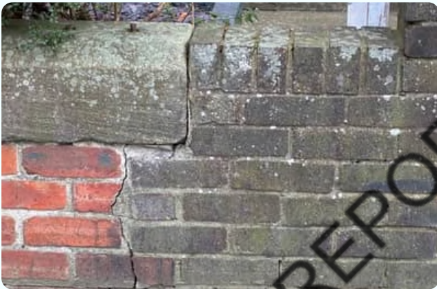
Moss and algae on brickwork
