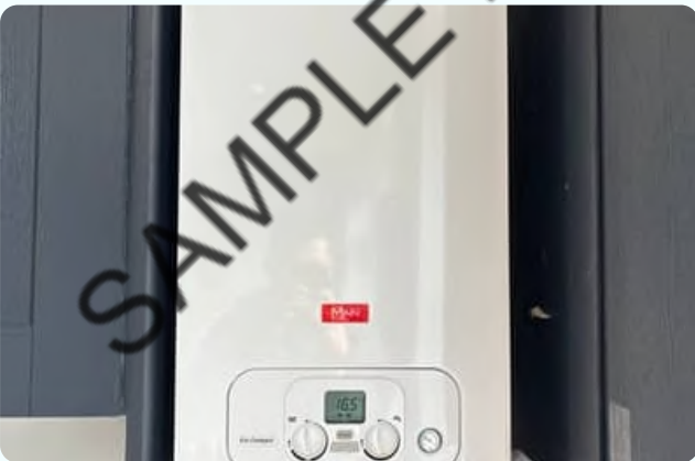
Boiler installed within cabinet
