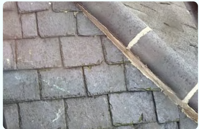
Moss and algae on roof tiles
