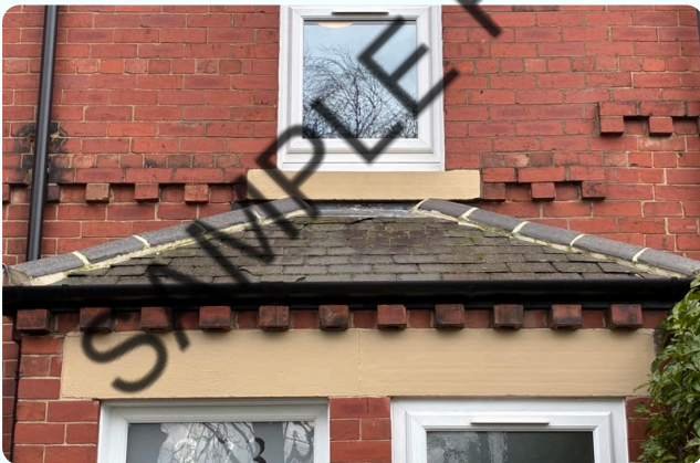
Moss and algae on roof tiles
