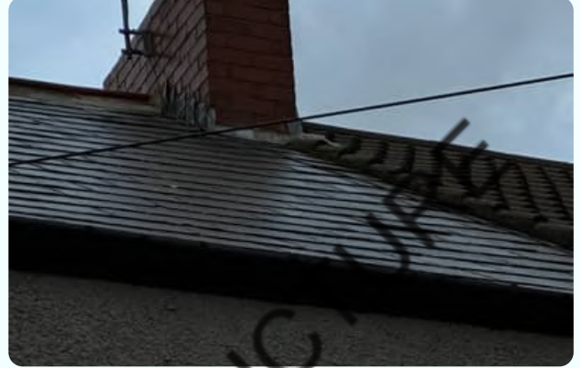
Flashing around chimney shows wear
