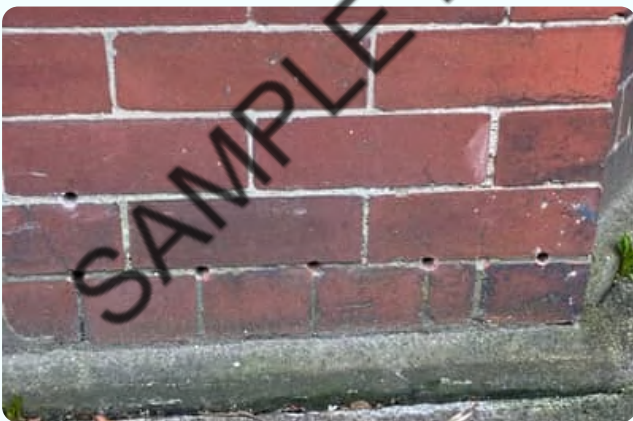
Damaged bricks and mortar loss
